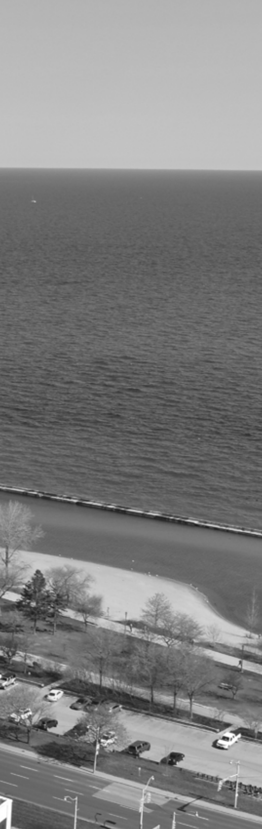
DIAMANTE URBAN CORPORATION'S MIRABELLA LUXURY CONDOMINIUMS UNDER CONSTRUCTION IN APRIL 2021 AT 1926 LAKESHORE BLVD. WEST, TORONTO. PHOTO CREDIT: SIWEI LI
